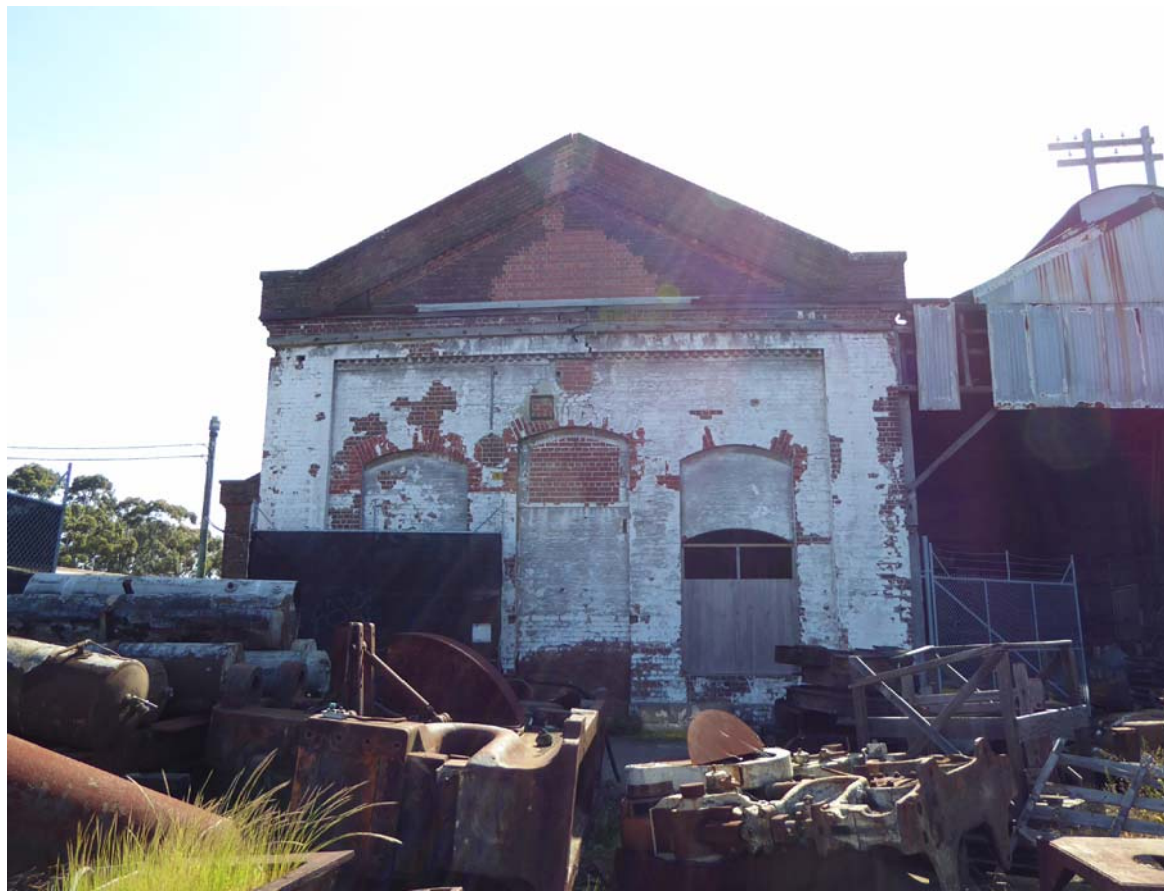
P-01 - WEST ENGINE ROOM
