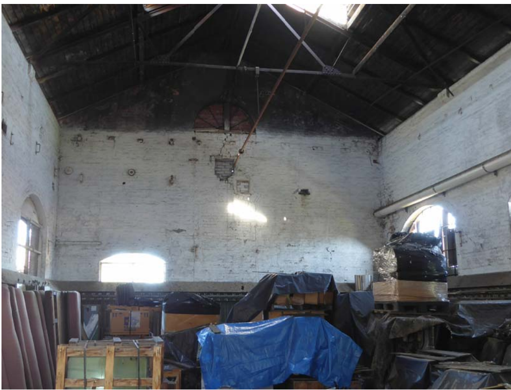
P-03 - WEST ENGINE ROOM (INTERNAL)
