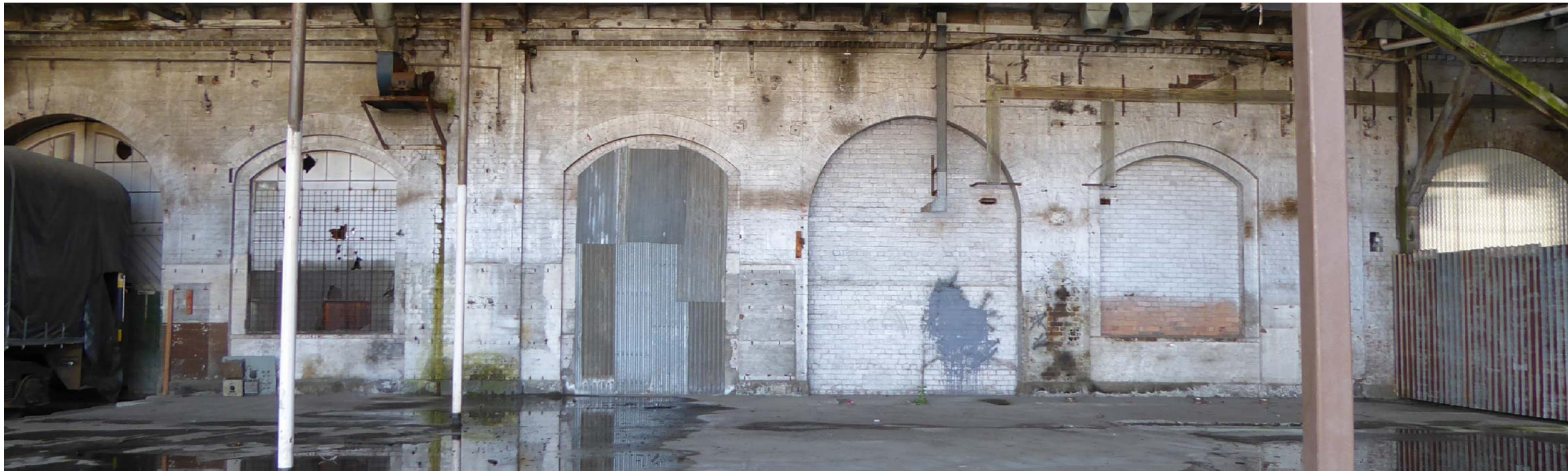
P-06 - AIR COMPRESSOR + WESTINGHOUSE BRAKE SHOP (INTERNAL)
