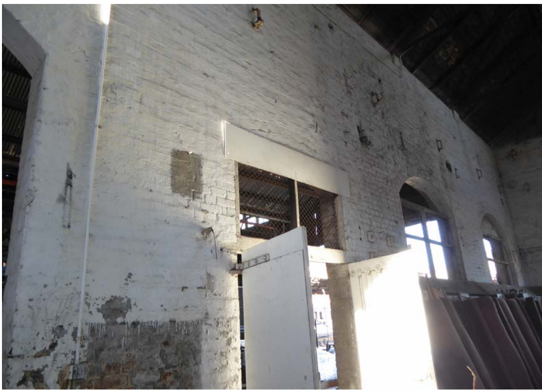
P-04 - WEST ENGINE ROOM (INTERNAL)
