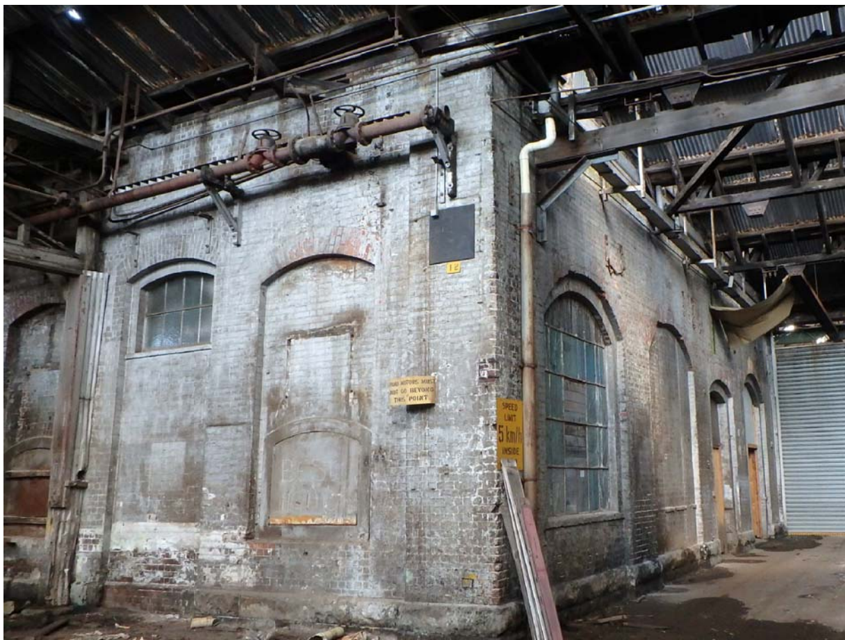
P-04 - EAST ENGINE ROOM
