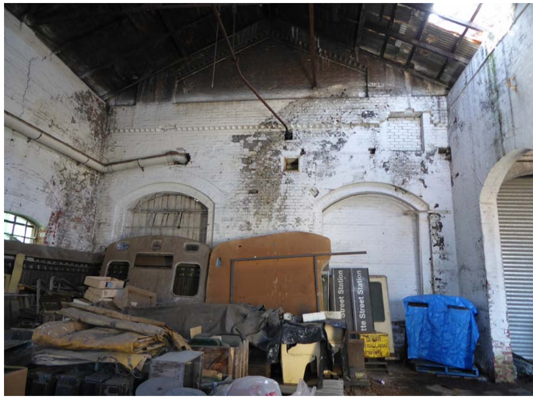
P-05 - WEST ENGINE ROOM (INTERNAL)
