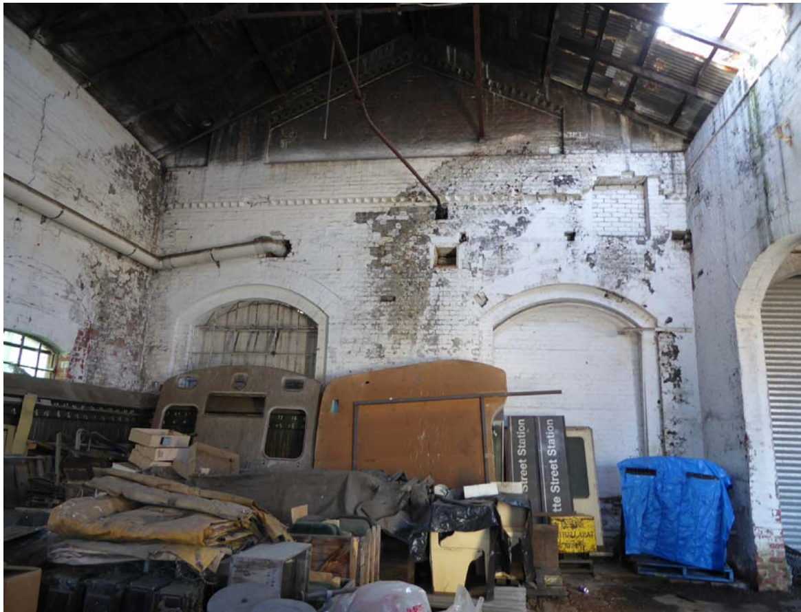
P-02 - WEST ENGINE ROOM (INTERNAL)
