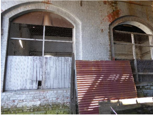
East side of West Engine House, showing paint finish and missing window frames
