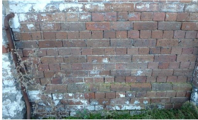
West Engine House, base of brick wall showing eroded mortar
