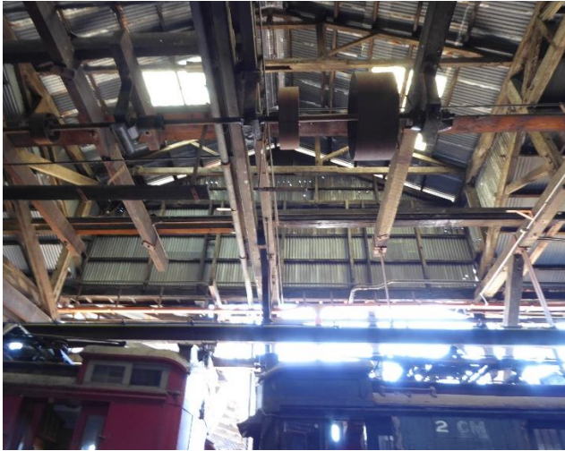
Line shaft belt and pulley system in Fitting Shop Extension
