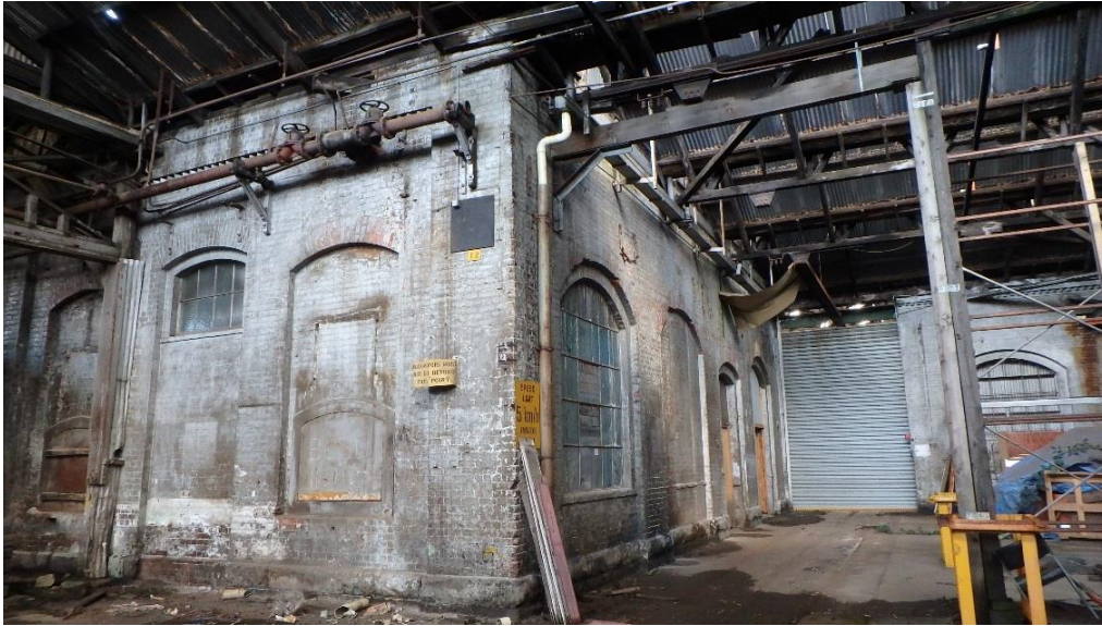
East Engine House, showing interface with the roof of Machine Shop Extension
