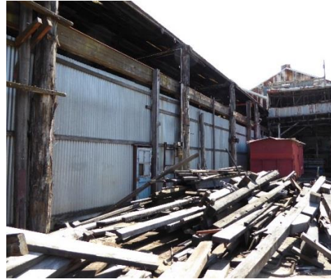
Boiler Shop Extension, east side, showing high sections of corrugated metal sheeting to walls
